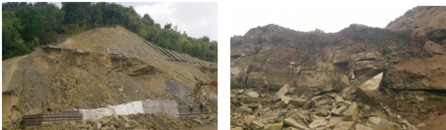
Figure 2. Slope Collapse and Landslide
