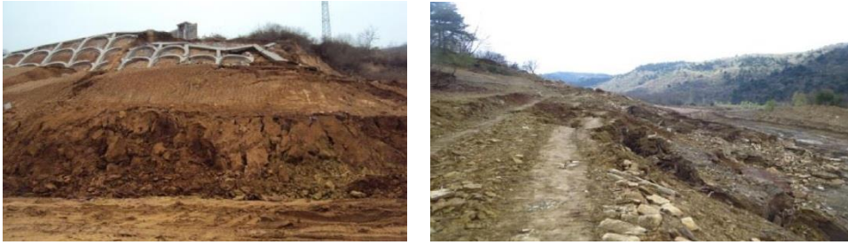
Figure 3. Slope Scattered and Collapse
