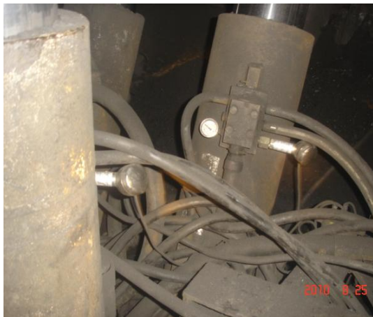
Figure 4b. Pressure Transducers fitted in the legs
