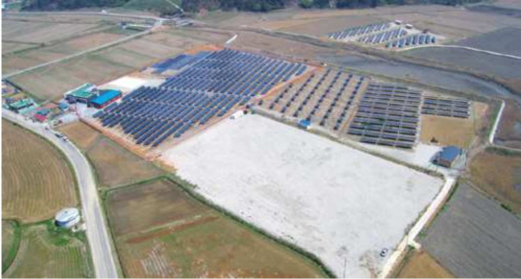
Figure 8. 1MW Solar Power Generation Demonstration Complex
