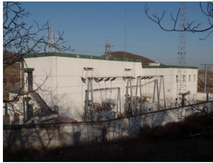
Figure 3. The Substation Physical Picture
