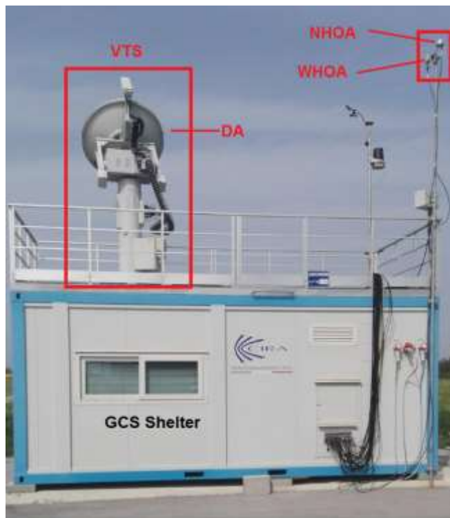
Figure 4. Ground Control Station with VTS, DA, WHOA and NHOA Antennas
