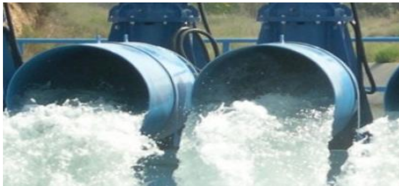
Figure 10. New Pumping Station in Manila City
