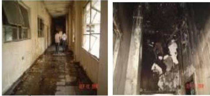
Figure 5. Fifth level hallway and portion of building affected by fire
