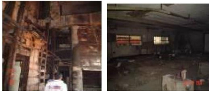
Figure 6. Portion of building affected by fire and inside the GSIS building
