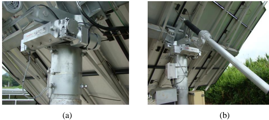
Figure 7. Operating Angle Sensor Driver Unit (A) Azimuth Driver (B) Elevation Driver
