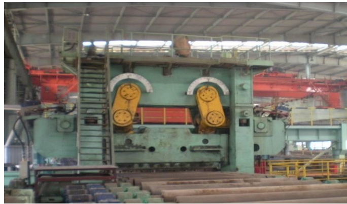
Figure 8. Picture of the Rolling Shear
