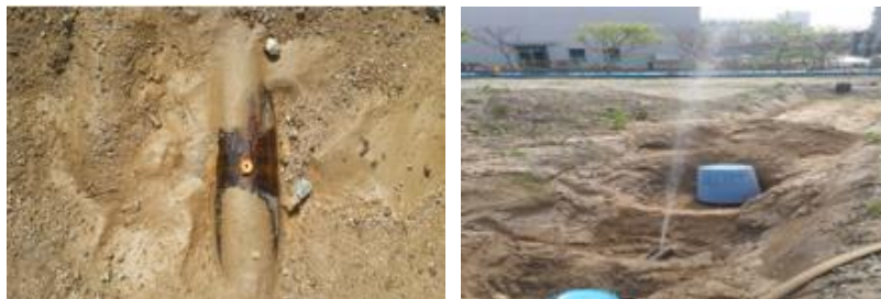
Figure 8. Leakage Hole and Water Leak
