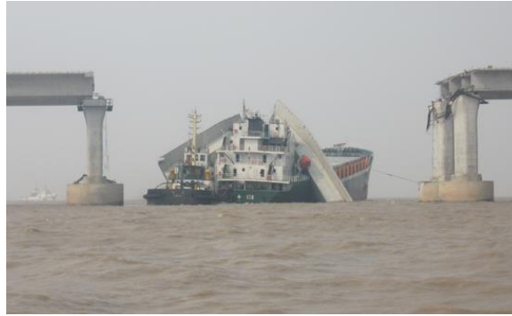
Figure 1. The JinTang Bridge in Ningbo Collapsed due to a Ship Collision
