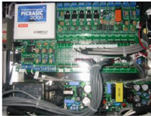
Figure 2. Control unit of DWCCS
