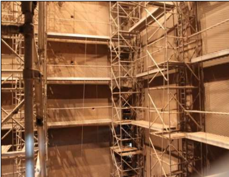
Figure 1. Power Plant Boiler
