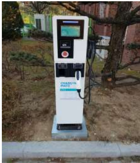
Figure 3. EV Charging Station in HNU
