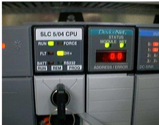
Figure 3. Allen Bradley SLC 5/04 Hardware
