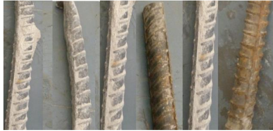
Figure 5. Shows Corrosion of Steel Bar Embedded in Reinforced Cement Concrete after 28 Days of Exposure
