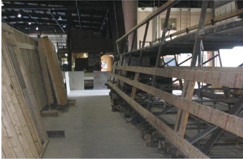
Figure 16. Framing, Piping, Electrical and Data Wiring and Sheet Rocking of Roof Truss
