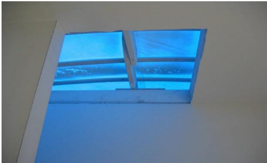
Figure 19. Roofs Covered with Plastic Material
