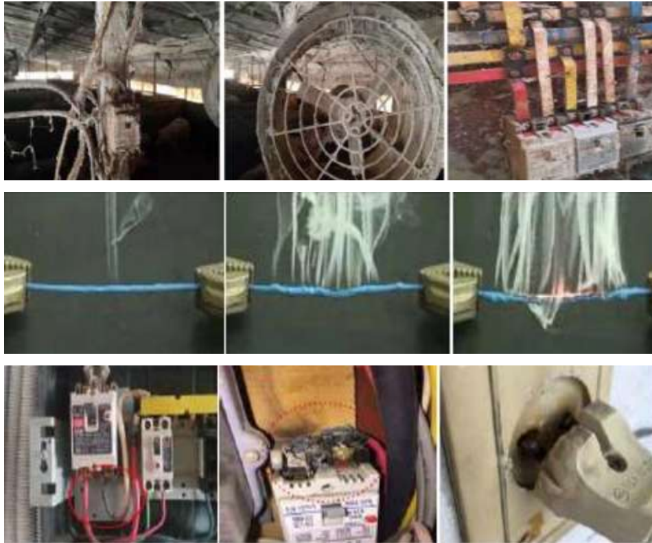
Figure 1. Poor Electrical Devices in Livestock House
