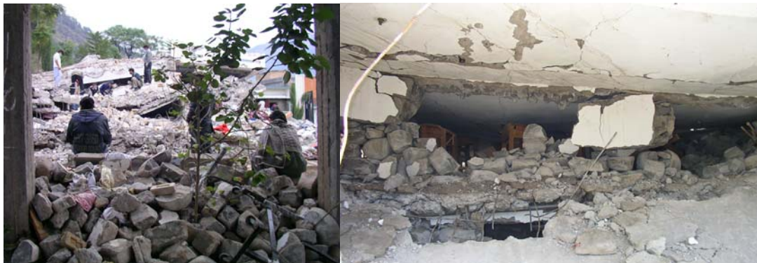
Figure 1. Pakistan earthquake 2005, locals attempting to search for survivors in a collapsed girl's college. The structure was in unstable condition; excavation and lifting machineries were prohibited from the site. (Pictures taken on site by author during mission)
